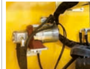
Emergency electric pump
